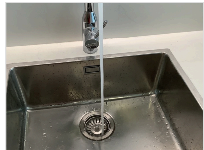
OK Kitchen tap and sink drain operating
