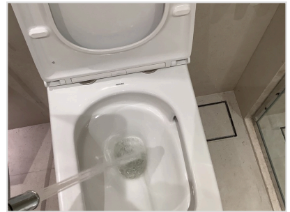
OK Toilet and bidet spray operating
