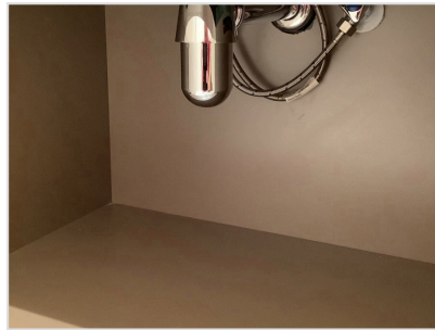
OK Basin drain operating
