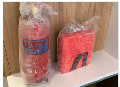
OK Entrance - fire extinguisher and fire blanket present
