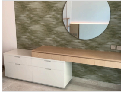
OK Dressing unit and cabinets checked
