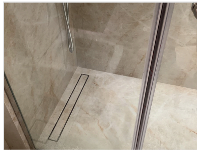
OK Shower drain operating
