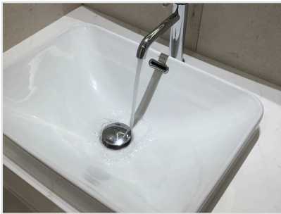
OK Basin and tap operating
